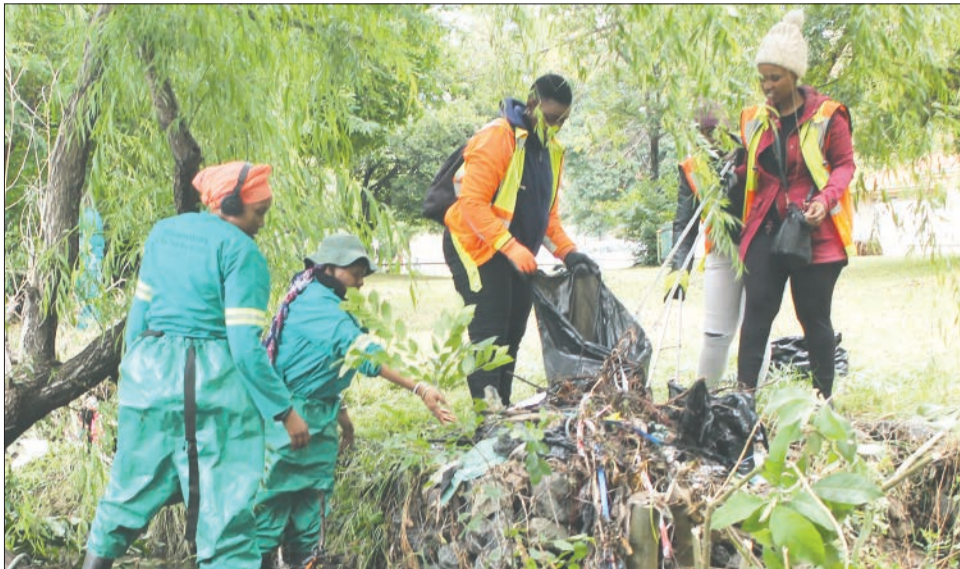
City Parks staff remove rubbish, standing on a tree that has blocked the spruit for years.
